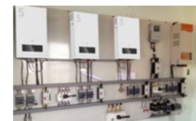
10 Salt Lake City, USA 2 MW Project Volume MPS-5K-48V-PLUS
